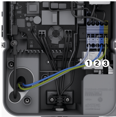
Fig. 14: Connection terminals (single-phase)
